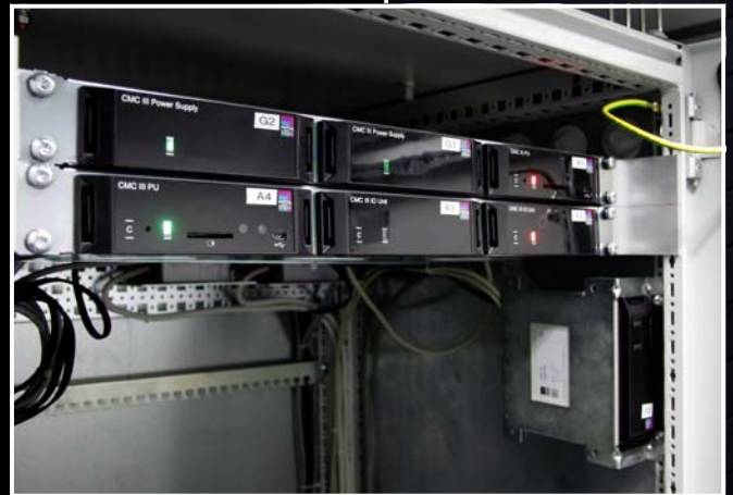
CMC III monitoring system
