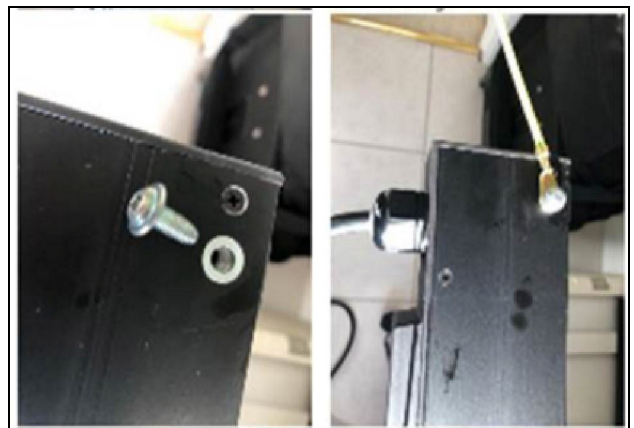
Fig. 15: Housing earthing point of the PDU
