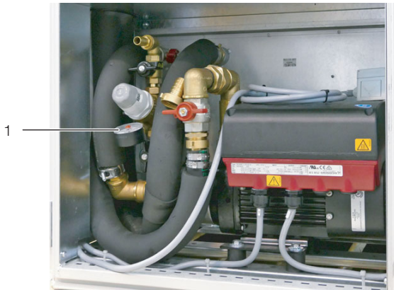
Fig. 44: Manometer in the water circuit
