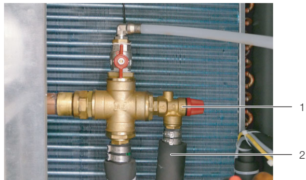
Fig. 24: Safety valve at rear
