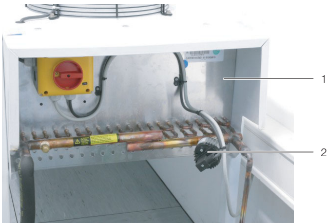
Fig. 27: Pressure switch on the condenser
