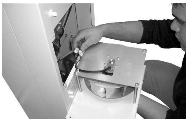
Fig. 69: Disconnect the fan connectors (1)
