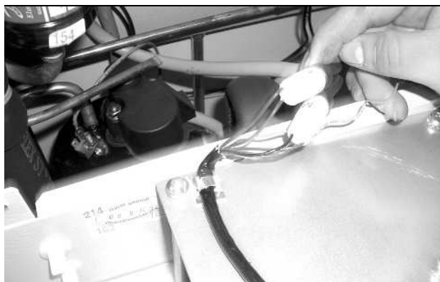
Fig. 70: Disconnect the fan connectors (2)
