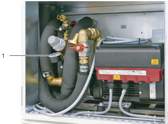
Fig. 48: Manometer in the water circuit
