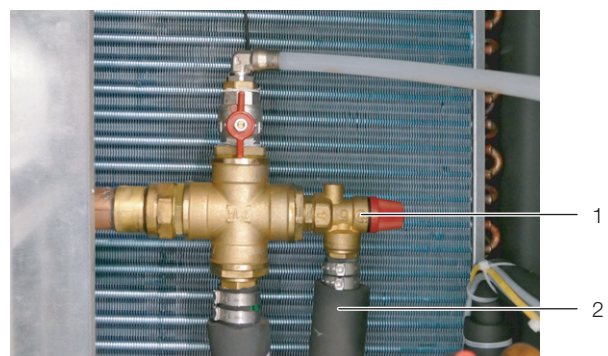
Fig. 27: Safety valve at rear
