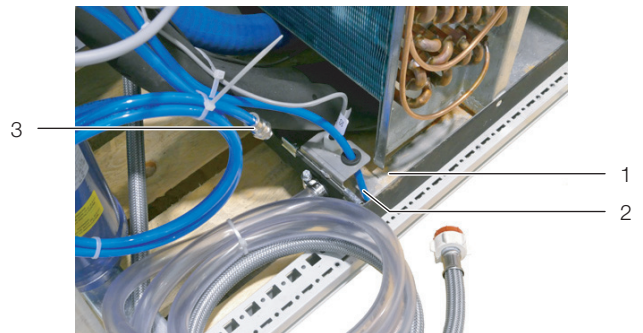
Fig. 63: Connections of the condensate pump
