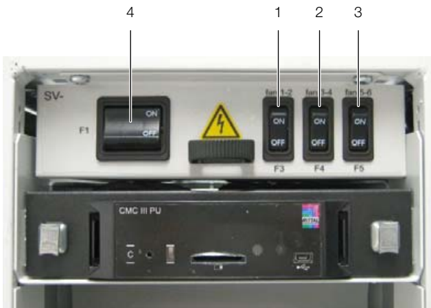
Fig. 29: Fuse box with master switch
