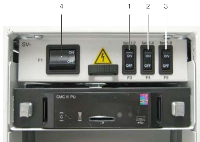
Fig. 13: Fuse box with master switch
